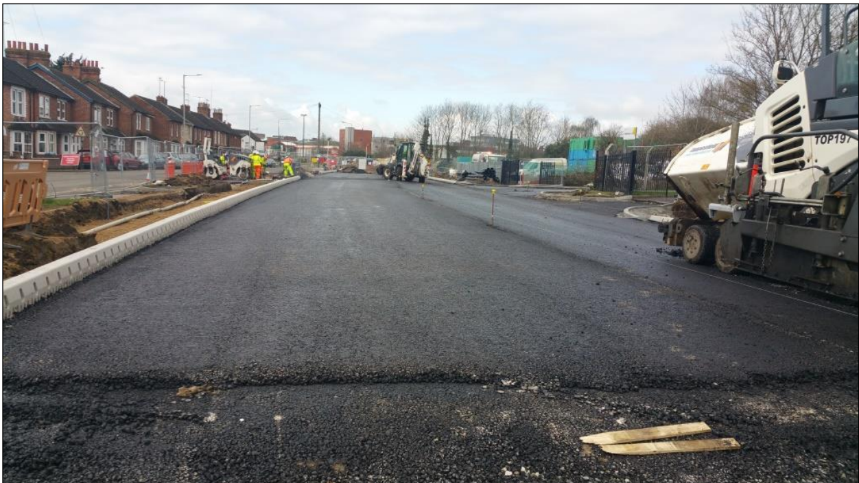
Kerbs installed and tarmac laid in Section 2 (in front of Stocklake Park School and Primrose Lodge access)
